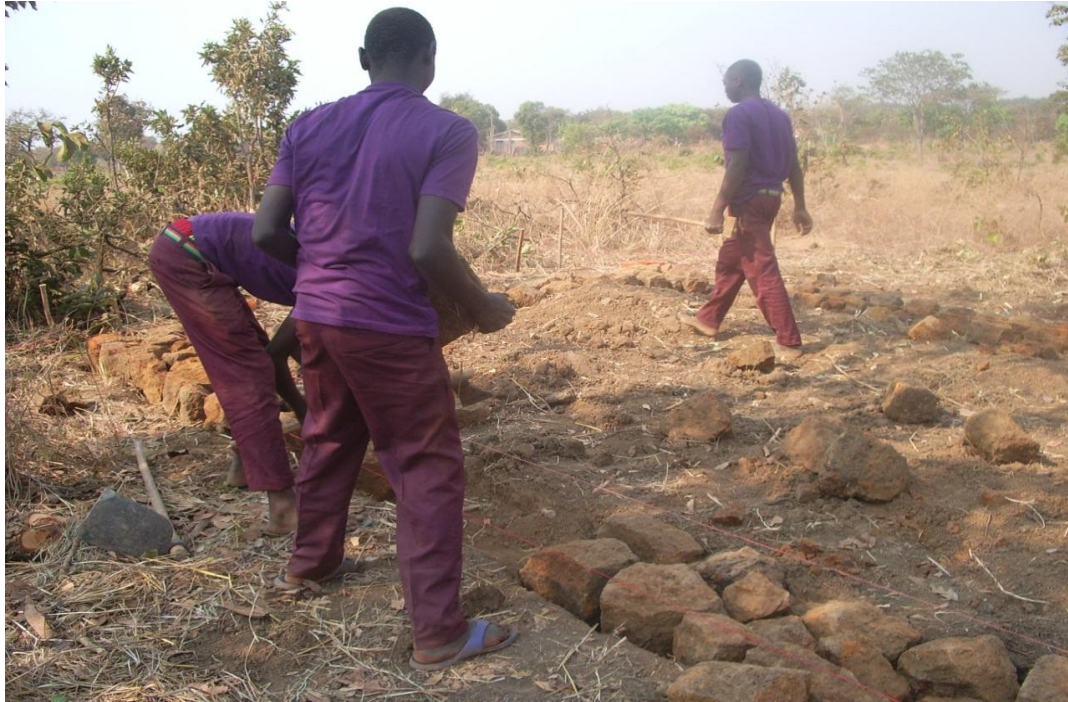
Figure 7: Youth on masonry department are now able to construct without a close supervision of their trainer. This picture shows Eliud Venance, Wilhad Bhulibha and Fredy Martin starting the construction of the house foundation in the village of Makere, on 24th December 2015- WEKEZA Program
